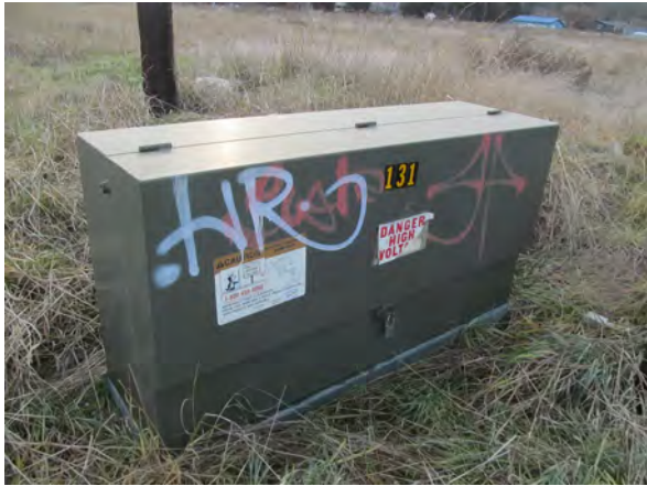
Photo #19 View of a pad-mounted electrical transformer on the northeastern portion of the subject property.
